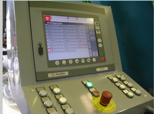
Touch screen controller
